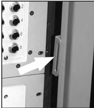
Figure 4. Cabinet door latch plate.
